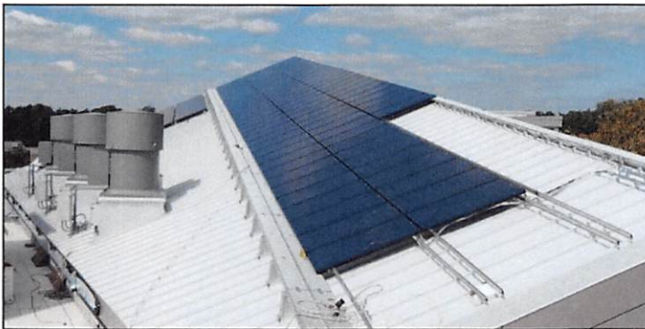
Rockville Campus Science Center Photovoltaic Array
