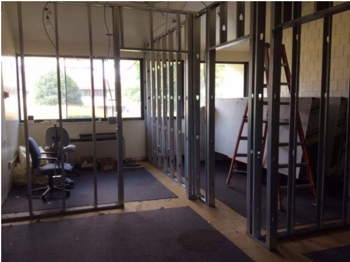
Germantown Campus—Science and Applied Studies Building Renovation - work in progress for ACES suite.
