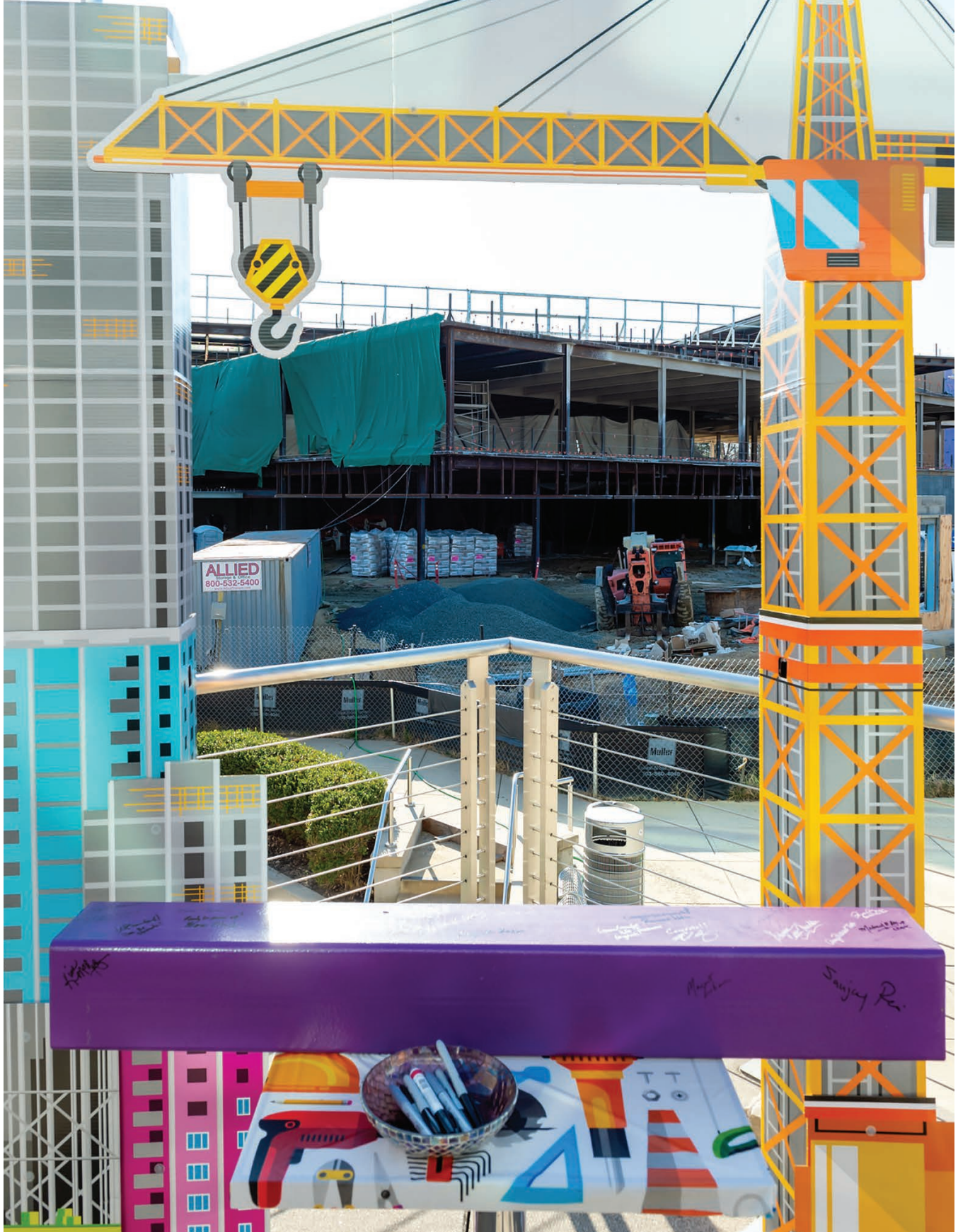
Construction progress continues on the Catherine and Isiah Leggett Math and Science Building on the Takoma Park/Silver Spring Campus. The 105-square-foot facility will prepare students for high-tech and in-demand career fields ranging from cybersecurity to life sciences. A ceremonial steel beam, pictured here, was signed by students, faculty, and staff on campus and presented to stakeholders at a ceremony in March.
